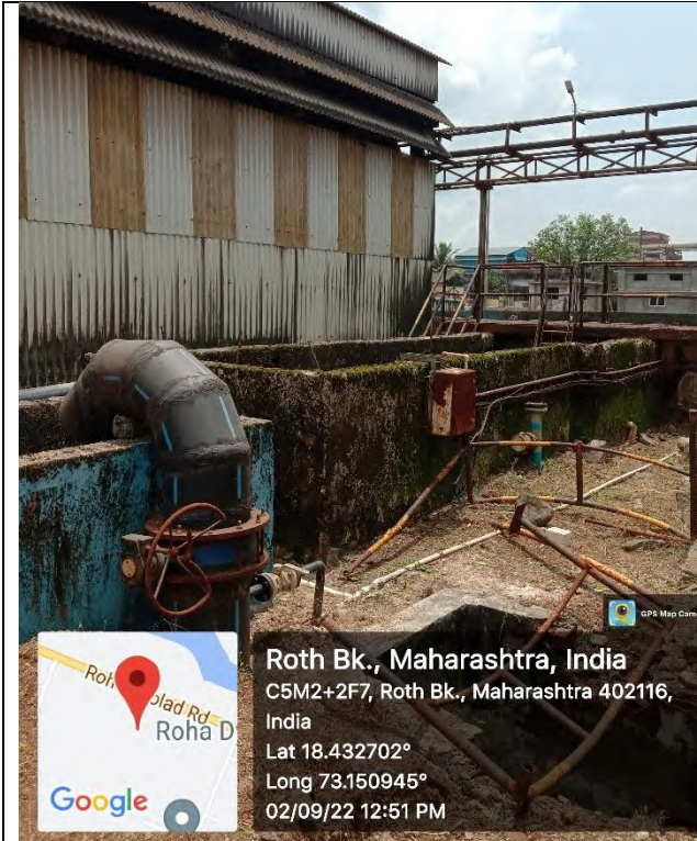
Photograph.1: Coarse Screen chamber
