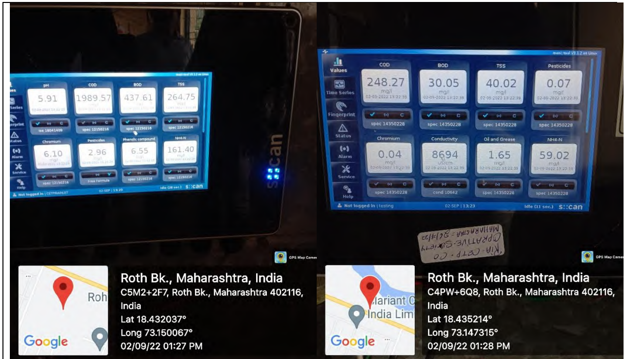
Photograph.13: OCEMS Panel- Inlet to CETP
